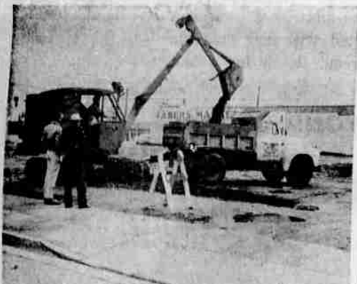
CONSTRUCTION UNDER WAY—Construction of the new First National Bank branch at Third and Pine sts. in Central Point began last week. A modern structure will be erected to replace the present branch at 136 Pine st. Meyers Jones Construction company of Medford was awarded the building contract on a low bid of $114,790.
