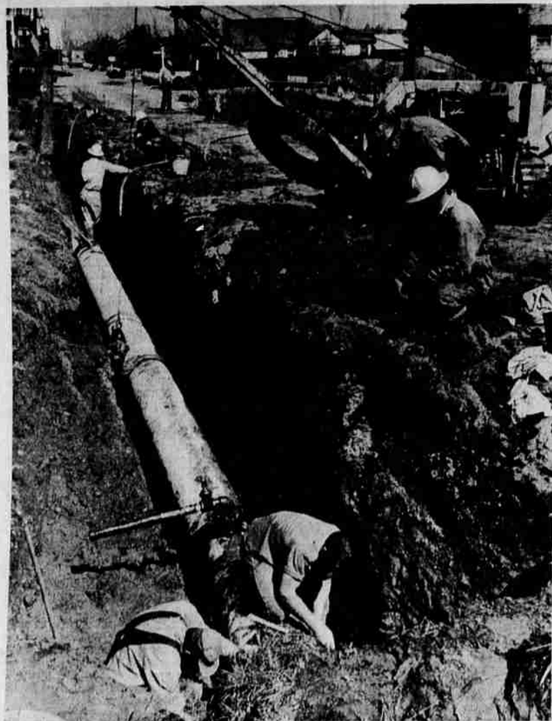
NEW MAIN —The new 24-inch water main in southwest Medford is expected to be in operation by July 1, according to Robert Lee, city water superintendent. The contract is for $239,484 and included 16,059 feet of 24-inch and 2,680 feet of 20-inch steel pipe plus related valves. Work started at the east end of Garfield st. and has progressed west to Columbus ave.
