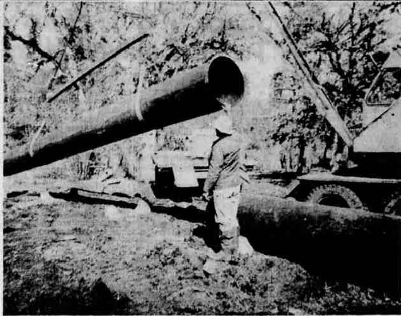
CONNECTING FLUME — Foreman C. J. Kelley of Eagle Point Irrigation is shown in place as repairs of a 2,000-foot flume near completion. The flume was washed out during the Dec. 2 flood.
