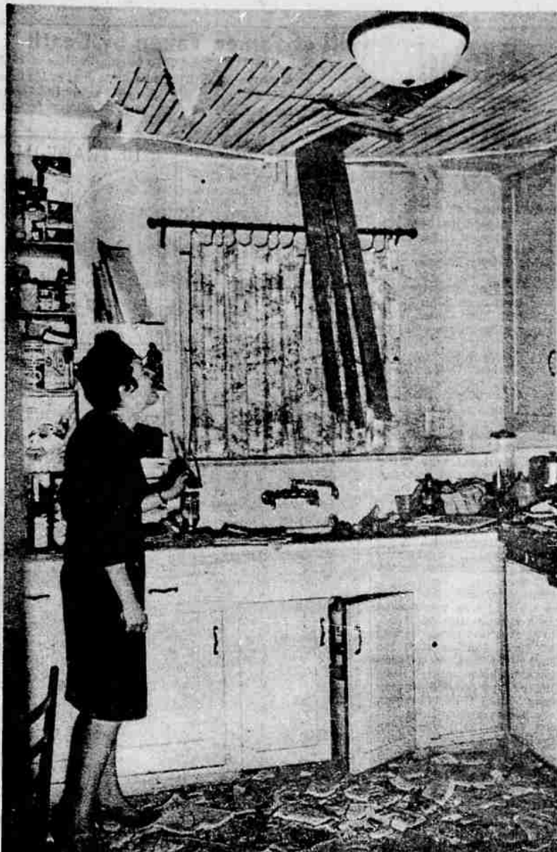
SMASHED THROUGH ROOF —Mrs. Erna Maurer looks up at wooden beam that toppled from a 22-story apartment construction site near her home in West Hollywood, Calif., Wednesday, and smashed through the roof, sending plaster cascading all over the kitchen. Mrs. Maurer left her kitchen sink to answer the telephone just seconds before the beam fell. (UPI)
