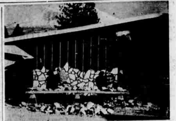
WORK COMPLETED—A group of masons from the Bill Warner company of Medford was responsible for construction of this rock work on the new student center building on the campus of the College of the Siskiyou at Weed. The building is due to be completed Feb. 28. The rock, material native to Siskiyou county, will also be used for fireplaces and other decorations in the building interior.
