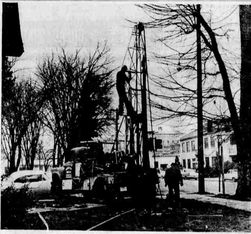
SOIL SAMPLES — Test holes to determine the type of footing necessary for Medford's new post office and federal building started this week at the site south of Library park. Five holes, ranging to 100 feet in depth, are being drilled by the Pittsburg Testing Laboratory, Portland. The picture above shows workmen operating the drilling rig at the corner of Eighth and Holly sts. this morning.
