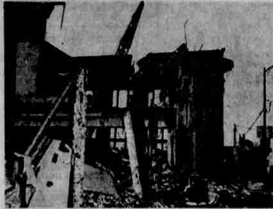
The proud old U. S. National Bank building in Grants Pass is gradually giving way to the efforts of Grants Pass wrecking contractor John Sims, but the battle still isn't over. Much of the 15-inch thick masonry walls are still standing.
