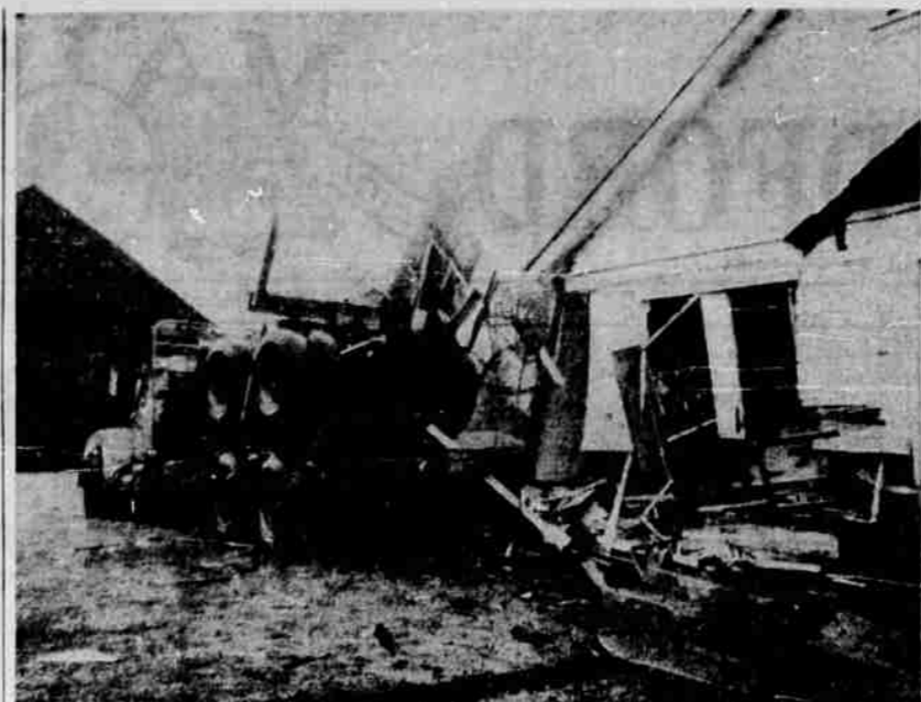
EXTENT OF DAMAGE — The front wall of the Peter Dee Flury home in the Prospect powerhouse area was torn out when a logging truck ran into it late Thursday night. There was heavy damage to the front bedroom, occupied by Peter Dee Flury, 31, and his wife Gwendolyn, 32. Both were taken to Rogue Valley hospital by ambulance.
