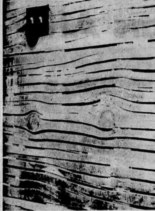
OLD WALL —The interior walls of the old house in Jacksonville were originally constructed in the manner pictured above. Flat boards were taken and sections of them were pruned and nailed up, after which plaster was stuck into the cracks.
