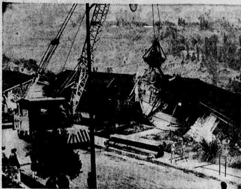
DAMAGED HOMES REMOVED —A wrecking crew starts work on removal of two homes damaged by an earth slide at Brentwood, Calif. The huge crane is demolishing the Henry Neel residence. The homes were first noticed moving Jan. 2 when the hillside behind them began slipping, wrecking several houses and threatening others. (UPI)
