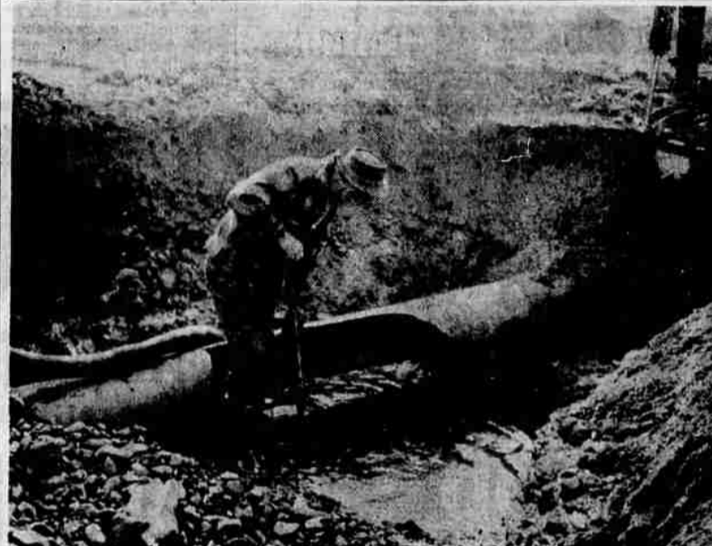
INSPECTS DAMAGE —Hubert Beer, construction foreman for the Medford water department, inspects damage to the 18-inch water main that crosses under Bear creek north of the Jackson st. bridge. The hole in the main occurred sometime during the Dec. 2 flood. Water department crews replaced the damaged section of pipe and the main was returned to service today.
