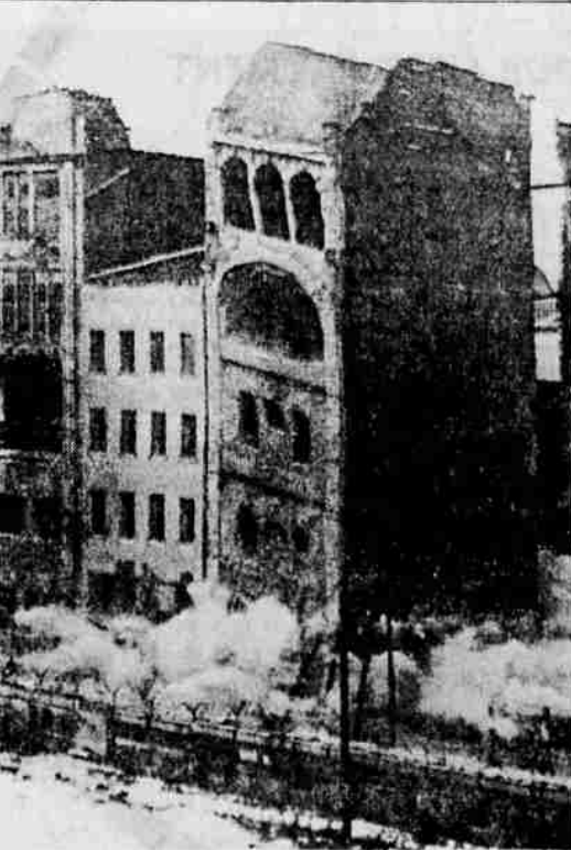
BUILDINGS DEMOLISHED - This view across the Berlin Wall shows clouds rising from explosions at houses along Zimmerstrasse in East Berlin, near U. S. "Checkpoint Charlie" as Communist police blow up the buildings to prevent use of their basements to conceal escape tunnels to the West, or as hiding places for refugees before escape attempts. (UPI)
