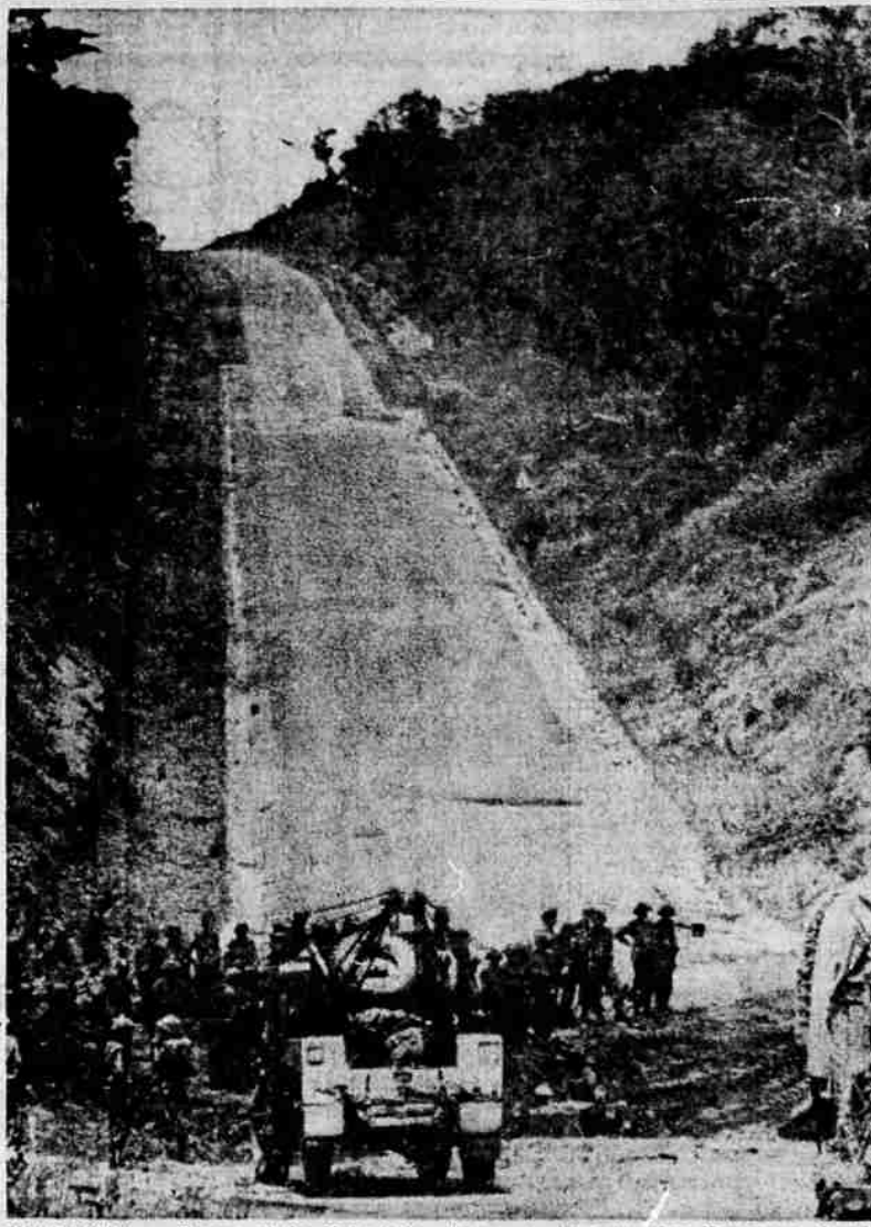
UN FORCES — Troops of the United Nations Fourth Madras (India) regiment are shown during the recent drive on Jadotville, which the UN captured Jan. 3. They are halted here near one of the bridges blown up by retreating Katangese. A soldier uses a bull dozer (half hidden in ditch, in foreground) to make the road passable for trucks. (UPI)
