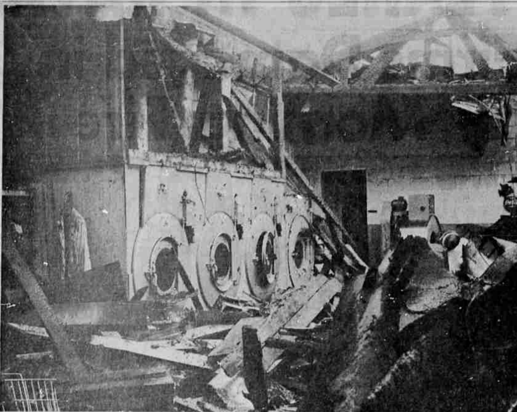
LAUNDRY—Four dryers along the north wall of the Big Y Laundromat are nearly buried in debris after fire swept the building Sunday morning damaging the laundry and three other firms. Owner of the firm, Raymond Niehaus, said that the majority of the equipment escaped fire damage, and that the loss was covered by insurance. The fire, believed to have started at the other end of the structure, spread through an attic. (Knackstedt photo)
