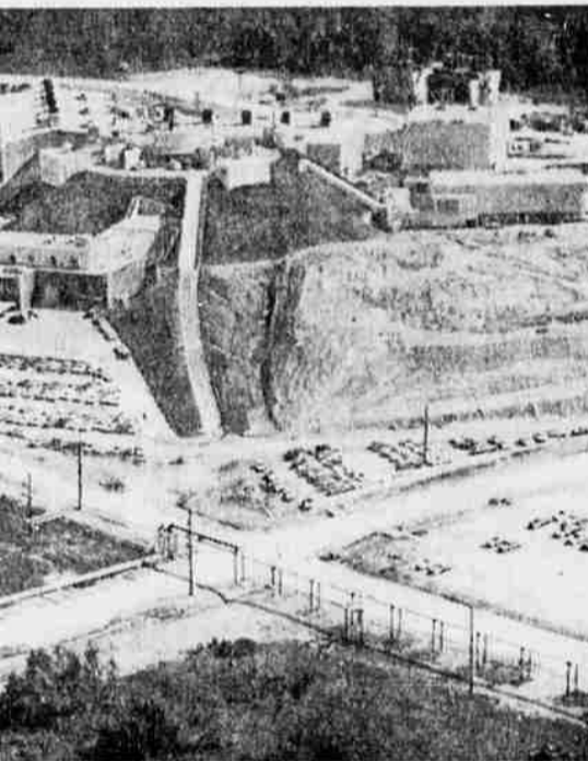
which sub-nuclear particles will be accelerated, will form the "heart" of the synchrotron. This magnet ring is being installed in an earth-covered structure in the center of the picture. At left is the framework for a high-energy physics research center. (UPI)
