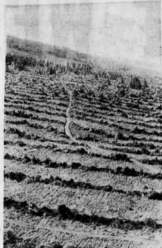
Service road breaks windrows of brush in the Cat Hill burn area where a tractor clears the land for replanting.
