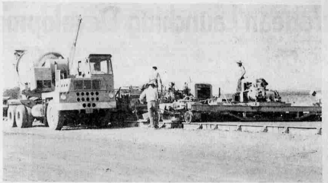
Equipment on rails, which serve as forms for concrete along the Freeway route, smooth and level concrete poured from large ready-mix vehicles. (Knackstedt photo)
