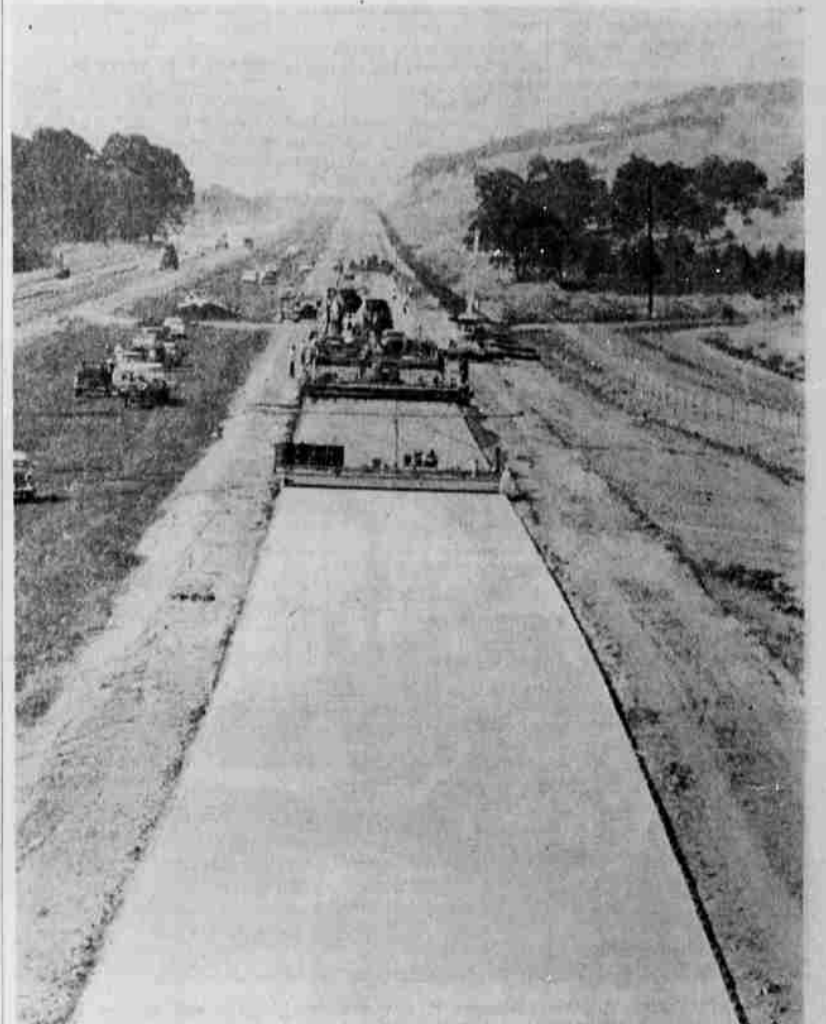
Laying a strip of concrete highway in the Phoenix area shown in this picture Freeway construction crews continued their northward progress recently.
