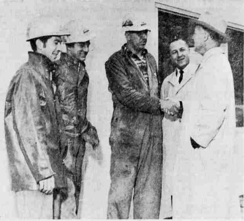
GREETs WORKERS —During his day of campaigning in Jackson county Tuesday, Oct. 9, Attorney General Robert Y. Thornton, right, spotted three men working on the remodeling of Landis Photo Studio and Severson's Candy store at the corner of Main and Grape sts. Thornton is seen here shaking hands with Bob Chriss while Oscar Privette, far left, and Louise Haussler look on. Standing between Chriss and Thornton is Alexander Diepenbrack, who was talking to the three workmen when the attorney general walked up.
