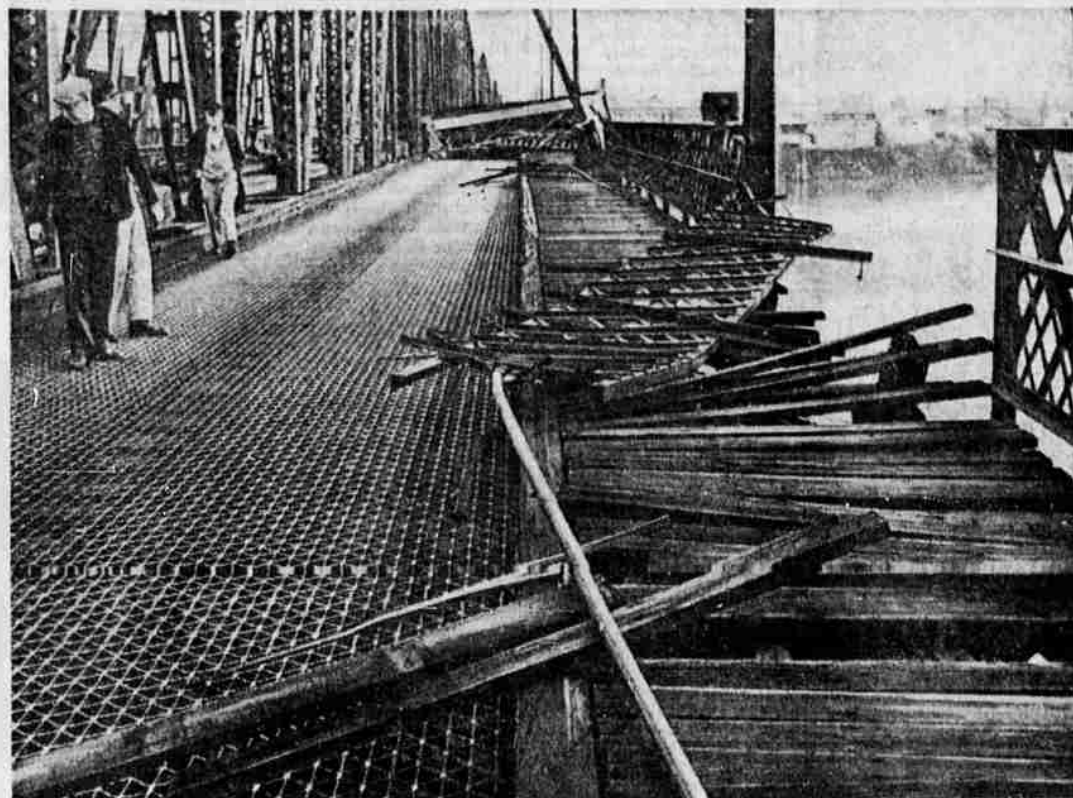
WALKWAYS DAMAGED — Metal decking on Hawthorne bridge in Portland and parts of wooden walkways were damaged by the storm Friday, making it necessary to close the bridge temporarily. — (UPI)
