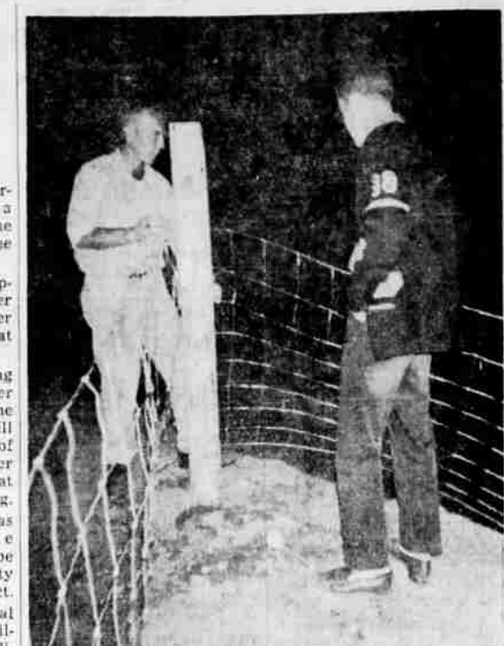
ERECT FENCE —Dr. Bruce Turner, left, and William Turner, members of the Central Point Junior Chamber of Commerce, are seen busy erecting the fence at Crater High School stadium recently. Like the Central Point Lions club, the jaycees contributed much time and effort to the stadium project.
