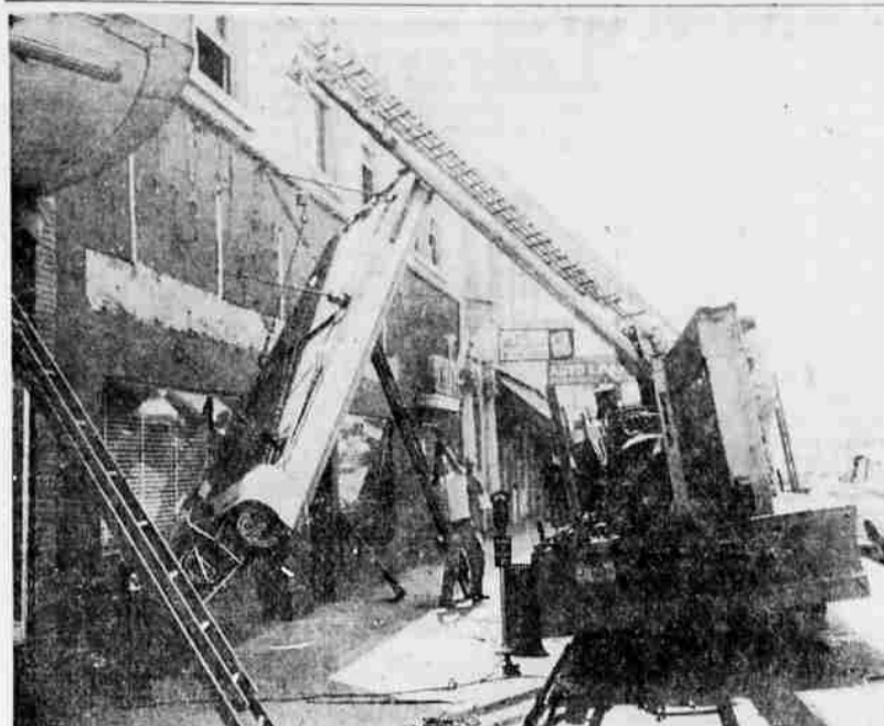
CANOPY REMOVED —Renovation work began this week at the former Top Notch cafe, 27 South Central ave., Medford. Stanley D. Smith, new owner of the restaurant, said only a little remodeling work would be done, especially to the exterior, before he opened Wednesday, Aug. 29. The restaurant will be primarily a fountain-lunch cafe, and will be known as the "Sip and
