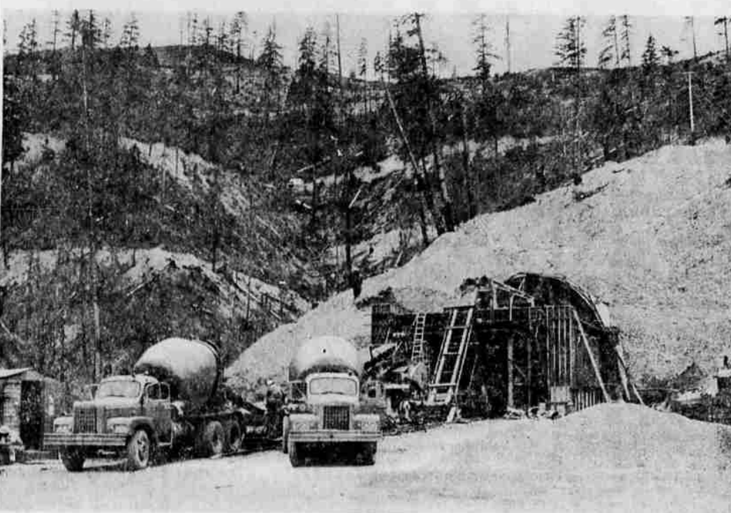
LINING—The Randolph Collier tunnel, which goes through Oregon mountain on Highway 199, is now being lined with concrete. The tunnel will eliminate a major bottleneck in the route to the coast. With the completion of the tunnel, the route to Crescent City, Calif., will provide the shortest and most direct route to the coast from Winnemucca, Nev. (Knackstedt photo)
