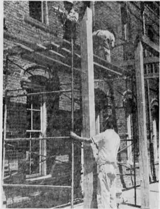
ERECT BALCONY —Orville Smith, contractor, puts some finishing touches on the balcony structure at the U. S. Hotel in Jacksonville. Assisting him is Alan Gallagher, Jacksonville. The balcony is modeled after the one which originally ran along two sides of the hotel on the second floor. The balcony was financed by last year's Jacksonville Jubilee. It is expected to be completed in time for this year's Jubilee Aug. 4-5.
