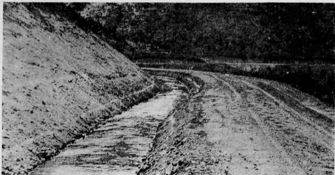
WEST CANAL —Water from Howard Prairie, Hyatt and Emigrant lakes streams through this irrigation canal along the side of the hills west of Talent to serve water users
