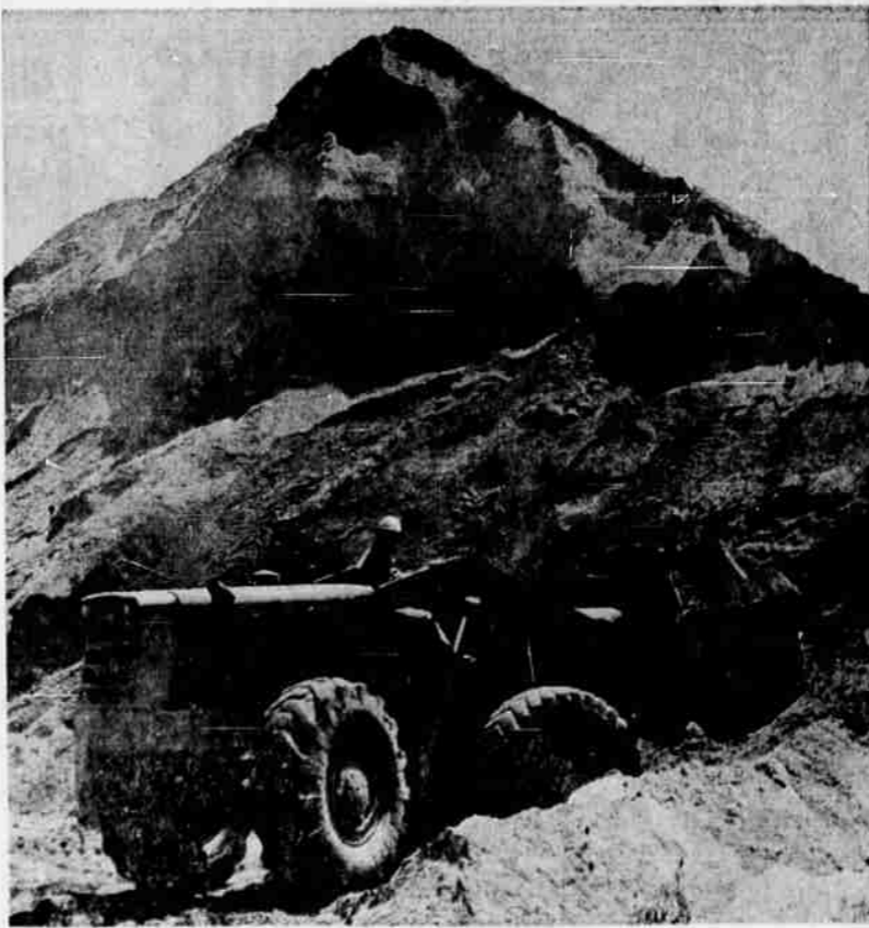
A front end loader feeds sand to conveyors at the batch plant. About 2,000 yards of concrete are being laid each day on the Seven Oaks-Jackson st. section of the Interstate 5 freeway.
