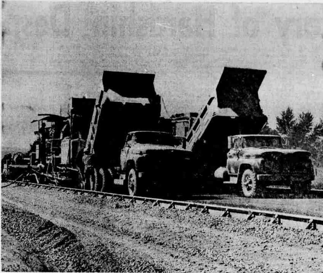
A fleet of trucks, hauling six yards at a time, keep the huge paving machine supplied with dry mix concrete. The paver has two mixing drums.
