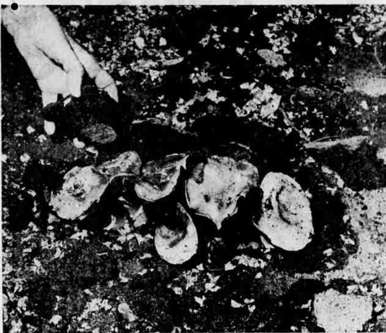
BUBBLE BURSTS — For several weeks this spring a bubble, which appeared in the asphalt pavement in the driveway of the Ralph Ellis home at 527 Putnam st., Medford, kept growing larger and larger. Finally, one day recently the bubble burst, disclosing six large mushrooms. Diameter of the larger mushrooms was estimated at four inches, and the stems "as big as broomsticks." What makes the natural phenomena even a little more unusual is that the asphalt, according to the Ellises, has been there for about eight years and this is the first time that growing material has appeared.
