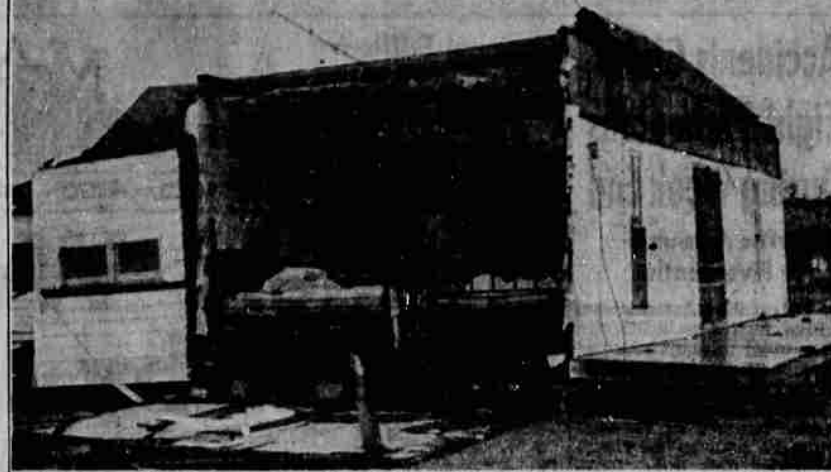
TORNADO DAMAGE — The side of this at Howe, Okla. The occupants were not in-house was neatly sliced off and the roof jured although the tornado left 15 dead and was carried away when a tornado struck 56 injured at Howe. (UPI Telephoto)
