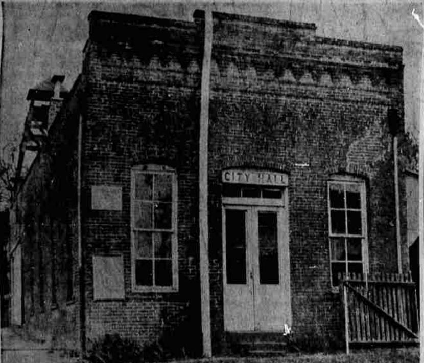
CITY HALL —The Jacksonville City council meets in the old city hall, first used as a general store in 1856. The council considers modern day problems in old style surroundings. The building is in need of repair today, and the city plans on soliciting bids for needed improvements.
