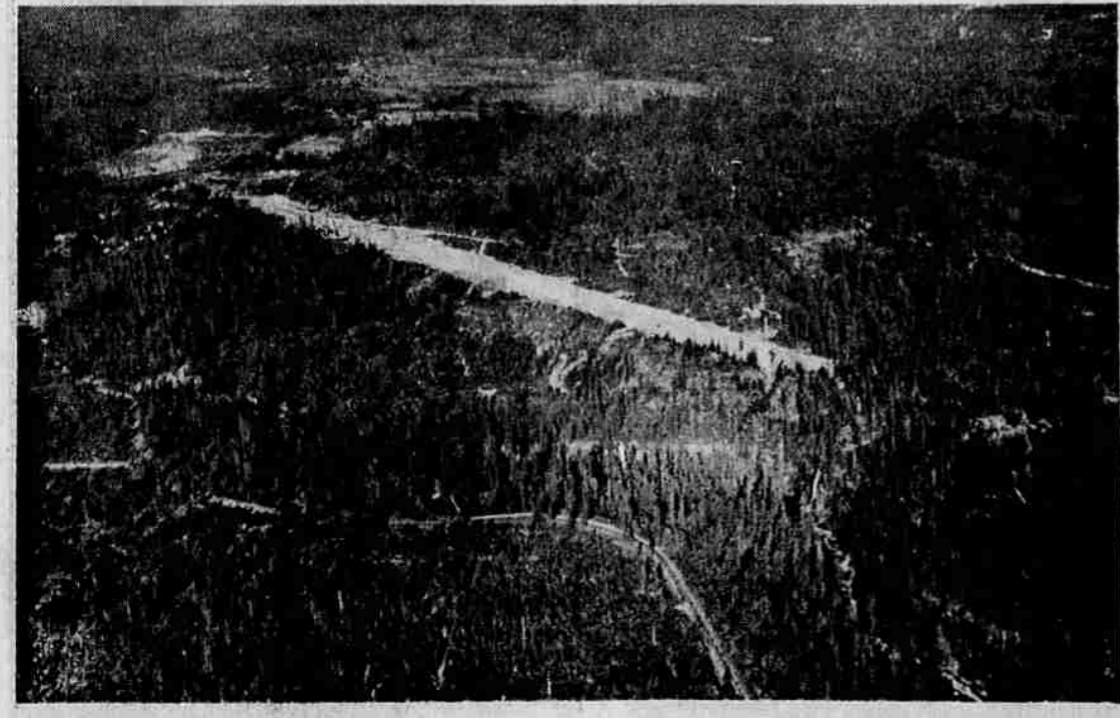
PROSPECT AIRPORT—Work on the Prospect airport is nearing completion. Construction started in the middle of January. The airport includes a 4,000 foot runway, with 1,000 foot approach clearings on the north and south ends. Surfaced width is 150 feet. Highway 62 is shown below the airport. Between the highway curve and the airport, the Mill Creek falls are visible.
