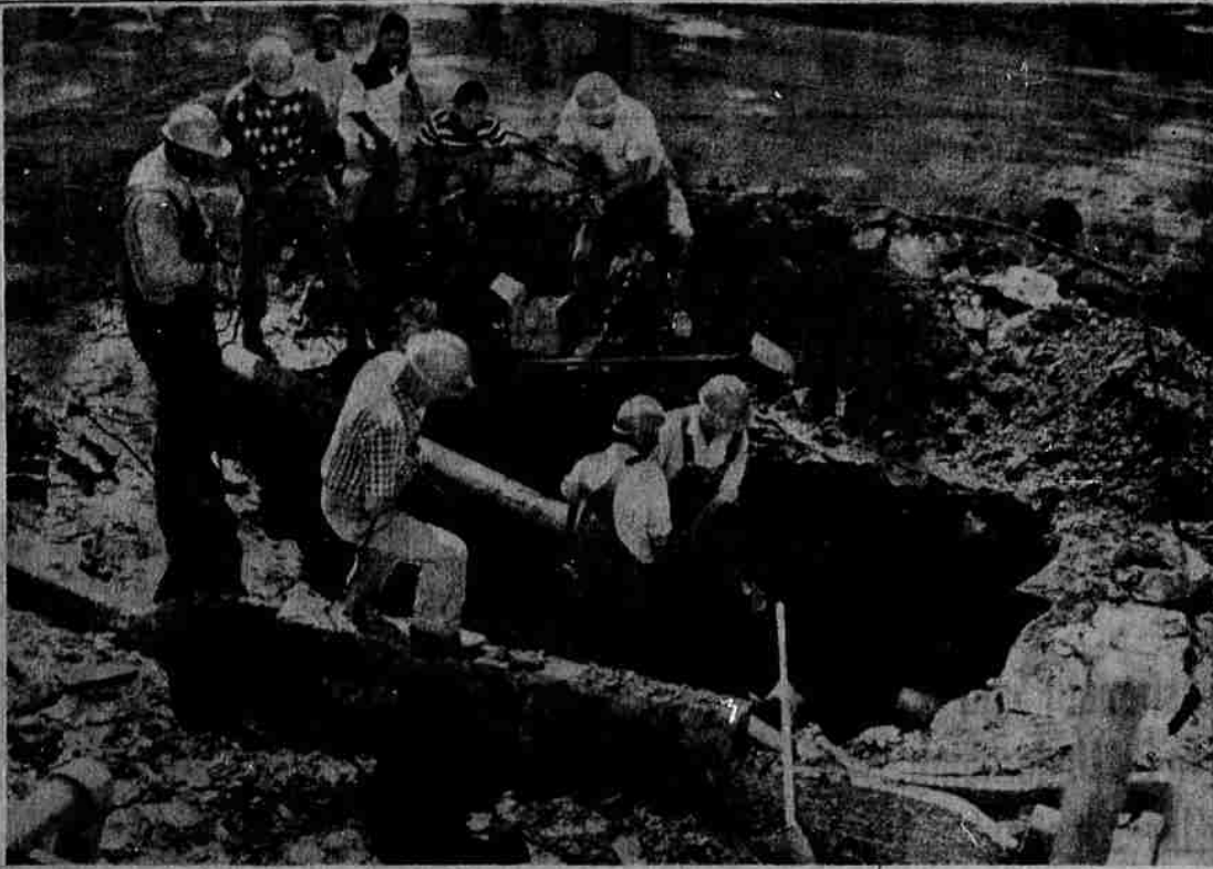
QUAKE BREAKS MAIN —Workmen repair a water main hit along the San Andreas Fault and jolted Hollister, 100 miles to the south, the hardest.
