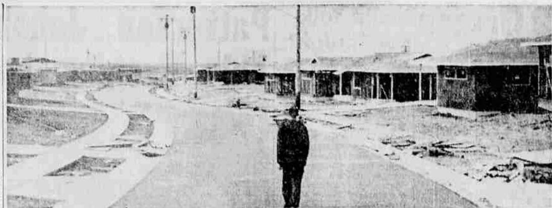
GHOST TOWN —The West's wildest ghost town is not Virginia City or anywhere near it. It's 12 miles from Marysville, Calif., on sprawling and strategic Beale Air Force base. Four hundred $16,500 homes, in all stages of construction, stand rotting along brand new but roped off streets. Construction of the project was halted last May 19 when the contractor encountered financing problems. Last month the U. S. Department of Defense said it would take charge of finishing the project with the Federal Housing Authority providing insurance funds. (UPI Telephoto)
