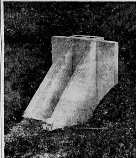
WASTE-WAY —This picture shows a concrete waste-way in the Talent lateral on the west side of the valley. Normally there are flashboard gates inserted in the box to control the outlet of water. This gate is opened to carry away storm or waste water in order to prevent flooding the lateral. The gate is left open to drain the lateral in the winter time when the irrigation water is not needed.
