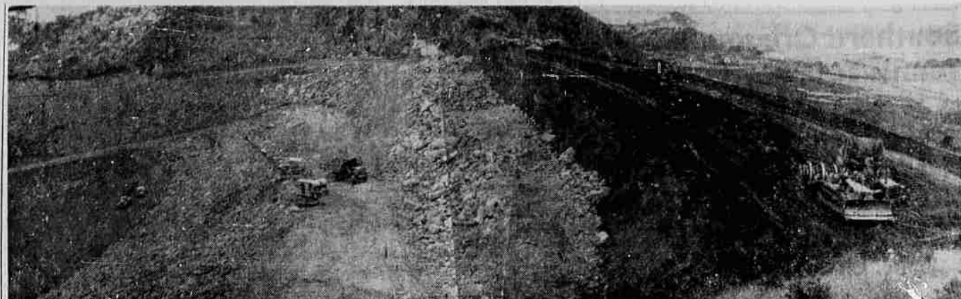
DAM ENLARGEMENT —This view shows the Emigrant dam enlargement. This is a composite picture showing the up-stream face. It is a view from the right bank near the axis of the dam. Contractor is R. A. Heintz Construction company. This dam is located on Emigrant creek east of Ashland. The dam is 196 feet high. The reservoir contains 50,000 acre feet. (F. E. Ross photo)
