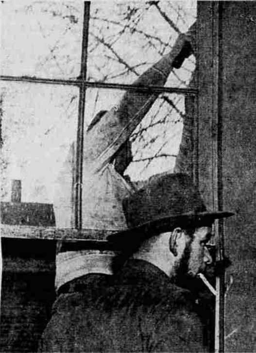
SCRAPE PAINT —George Brewer and Norman Butts, both of Jacksonville, scrape at some of the old blistered paint around a window frame in the pioneer U.S. hotel. Work parties have been at the hotel almost every day scraping paint, hammering, sawing and generally cleaning up the pioneer landmark. The people working on the hotel need donations of money and materials, but particularly need more manpower to continue the work.
