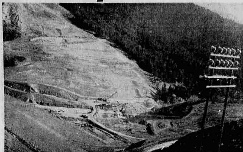
NEARING COMPLETION - The final load of clay was placed and packed into place in the Trinity river dam in northern California recently. This picture shows the dam, at lower left, nearing completion. It was
