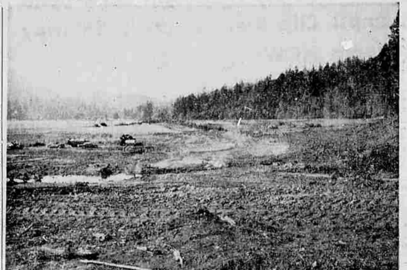
UNDER CONSTRUCTION—McMullen creek reservoir near Selma is being built by the Josephine county court in cooperation with its parks department. The 156-acre lake will be used for warm water fishing and many other recreational activities.
