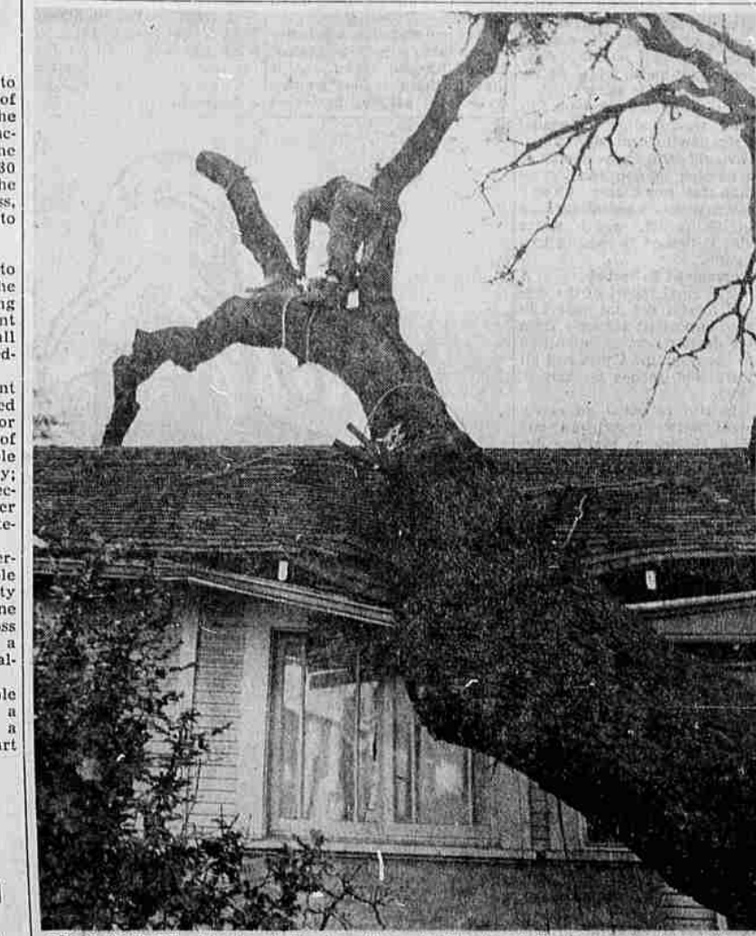
REMOVE TREE—Linebaugh Brothers Tree Service crews yesterday removed this white oak tree from the roof of the home owned by Gertha Lane, 714 South Oakdale ave., Medford. The tree, estimated by Linebaugh Brothers to be about 400 years old, fell across the house roof, damaging the roof, wall and windows. The tree had been leaning for some time, and broke off at the ground.
