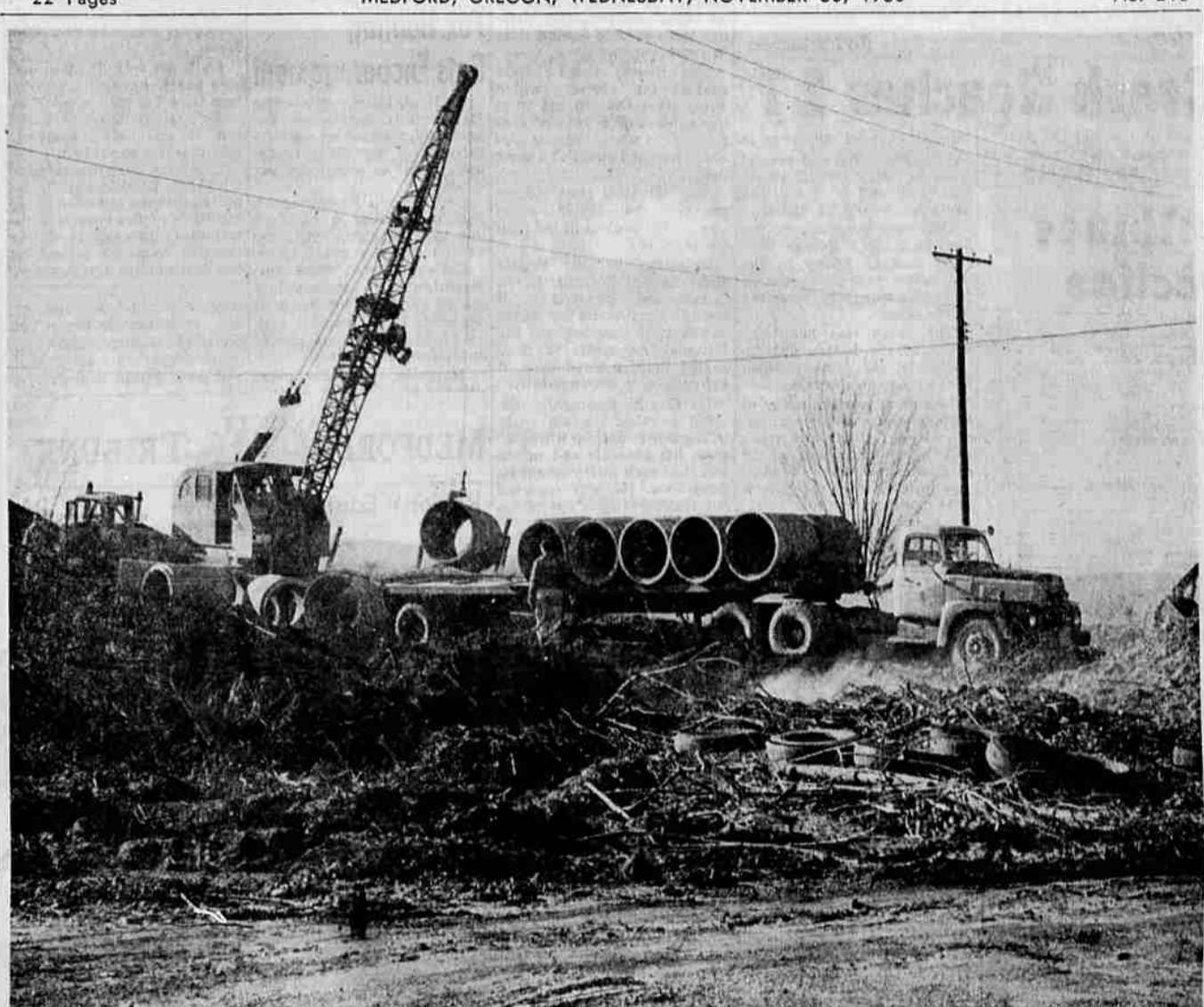
BIG TILE —At the point where new Highway 99 freeway will cross Table Rock rd., some 475 feet of 36-inch concrete tile is currently being laid as a passageway for a 6-inch water main. According to Clay Sugg, foreman of the project, the tile will allow water to escape in the event there is any leakage from the main, thus preventing undermining or softening of the M. C. Lininger and Sons, Medford, are contractors for the job.
