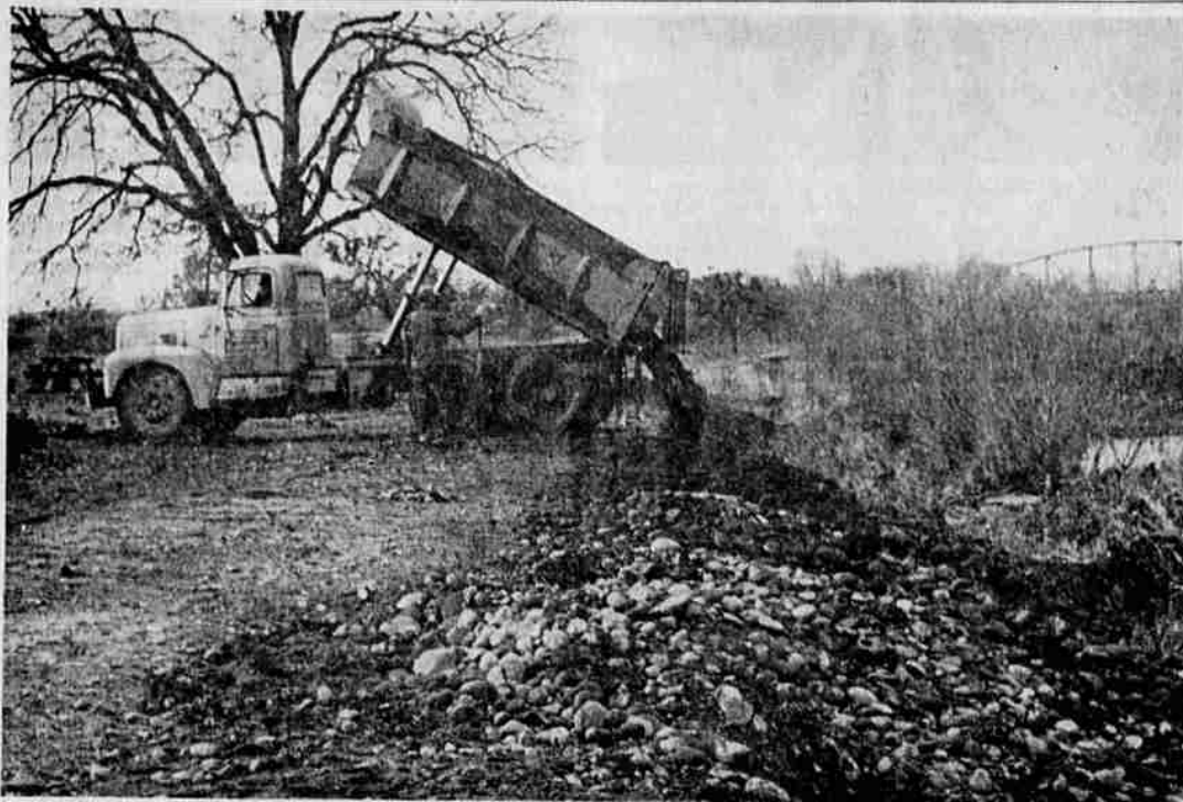
RIP RAP—In order to prevent erosion to the east bank of the Rogue river that runs along TouVelle State park, some 500 yards of rock and gravel are being used to cover the sandy soil at the river's edge. During heavy runoff periods, the water running through the channel between the island and the park has been cutting into the bank because of the turn it makes to re-join the main body of the river. The picture above, taken this morning, shows a truck dumping its load, while Carl Bennett, state parks division employee, oversees the job.
