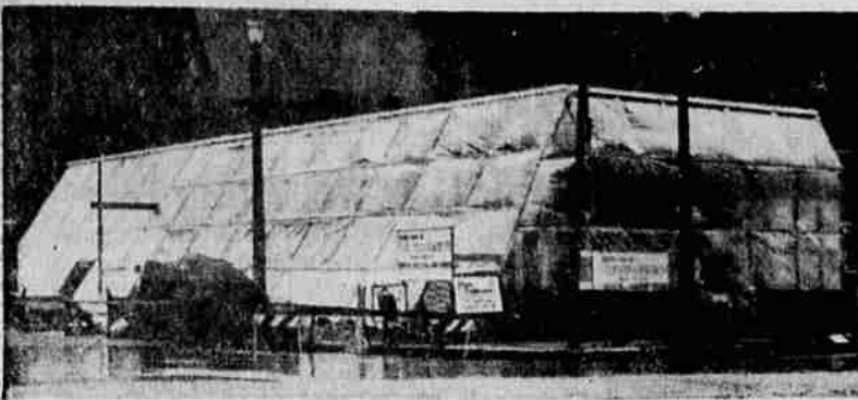
CONSTRUCTION GOES ON - Faced with a Jan. 1, 1981, deadline at which time a state granted charter expires, the contractor hired to build a new St. Louis, Mo., bank completely encased the two-story structure in plastic. The covering allows workmen to construct the outside walls regardless of the weather. The area under the plastic can be heated if necessary to aid in drying paint, cement, etc. (UPI Telephoto)
