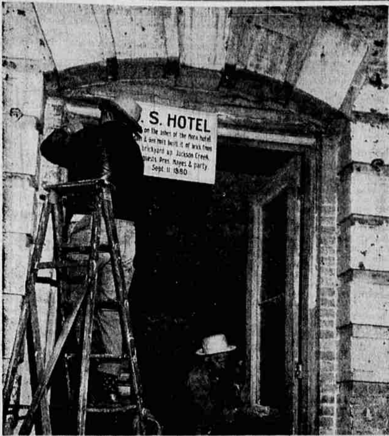
RESTORATION UNDER WAY —Ex-miner J. O. Morgan, 1021 South Third st., Ashland, was one of the first volunteers to begin work Tuesday on restoration of the U.S. hotel in Jacksonville. He is shown scraping paint from the hotel main entrance. Ernie Dorn, 400 D st., Jacksonville, also scraping paint, is another of the many volunteers expected to help with restoring the historic old building which was once the center of social events in the gold town of Jacksonville.
