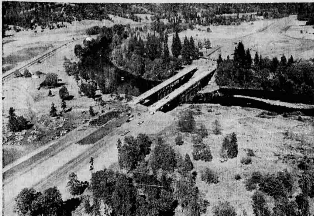
FREEWAY WORK — The Highway 99 Freeway bridge across Rogue river near Homestead on the Rogue north of Gold Hill is reaching the completion stage by Pacific Concrete company, Portland. During the construction period, 110-foot booms were used to pour concrete, and two local transit mix companies joined to keep concrete moving to the location. An overpass over the present Highway 99 (at the far end of the bridge above) has been started. —(Whitland Locke Photo)
