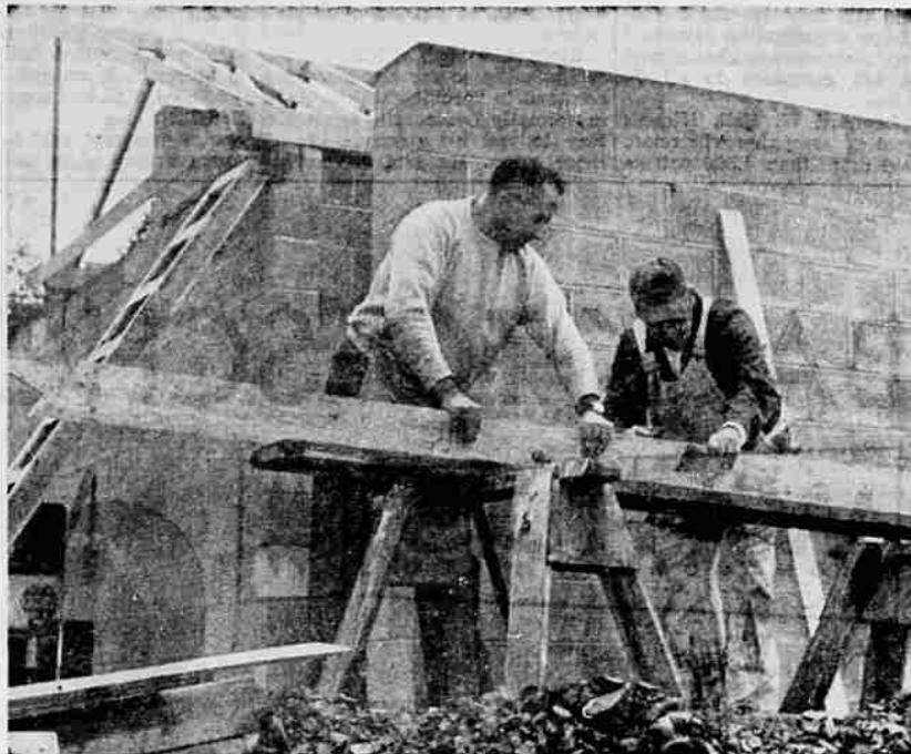
COMPLETING RESTROOM —Bert Marshall, Central Point, and Jim McGowan, Medford, were preparing timbers for the roof of the rest room of concrete block at the Hooper Springs recreation area off Dead Indian rd. The picture was taken last week as the men rushed work on the building in time to catch the last of the summer season tourists en route to Howard Prairie reservoir.
