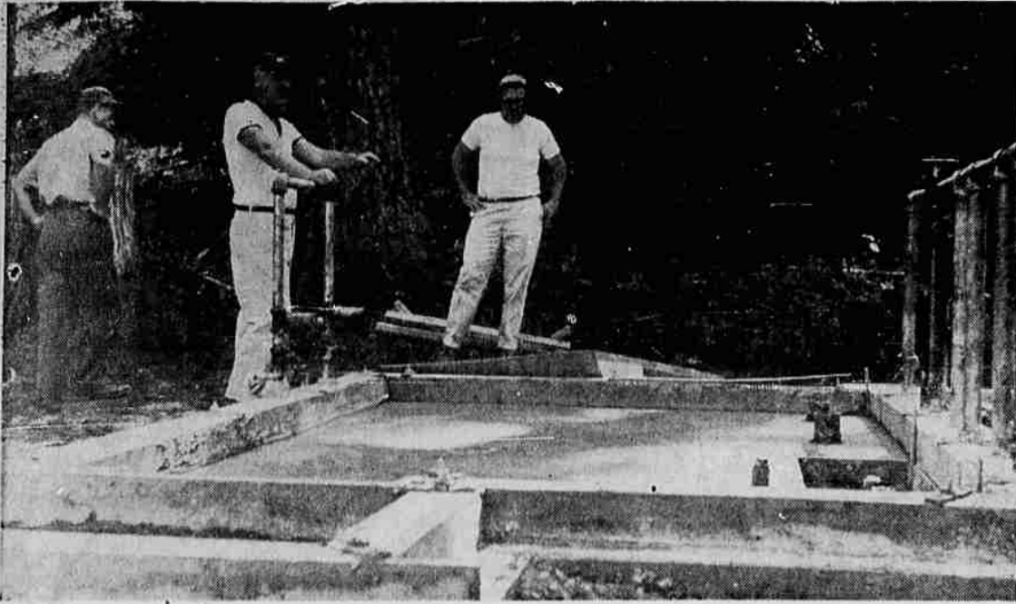
BEST ROOM FACILITIES —Bob Johnston, manager of Johnston Stores, Medford, concessionaire at Howard Prairie reservoir, (left) and Robert Haworth, city-county parks and recreation director, examine the foundation and basic plumbing of one of the restroom facilities being constructed at Howard Prairie reservoir. At extreme left with his back to the camera is Sid Wilkinson, Medford resident.
