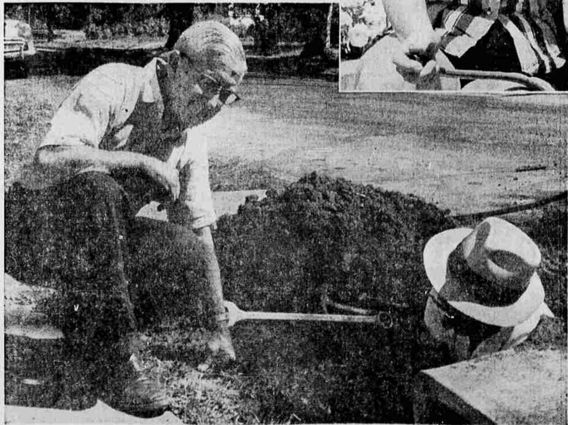
Doing a little "sidewalk supervising" and picking up a few pointers while a city crew installed a water meter on Crater Lake avenue Wednesday morning was nearby resident W. E. Halbrook, at left. Working on the meter is water department employee Hubert Beer.
