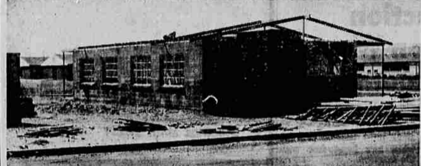
JEWETT ADDITION — Included in the school additions in district 6C, which includes Central Point, Gold Hill and Sams Valley, is this addition to Jewett school. The addition is expected to be ready this fall to handle an increased number of students.
