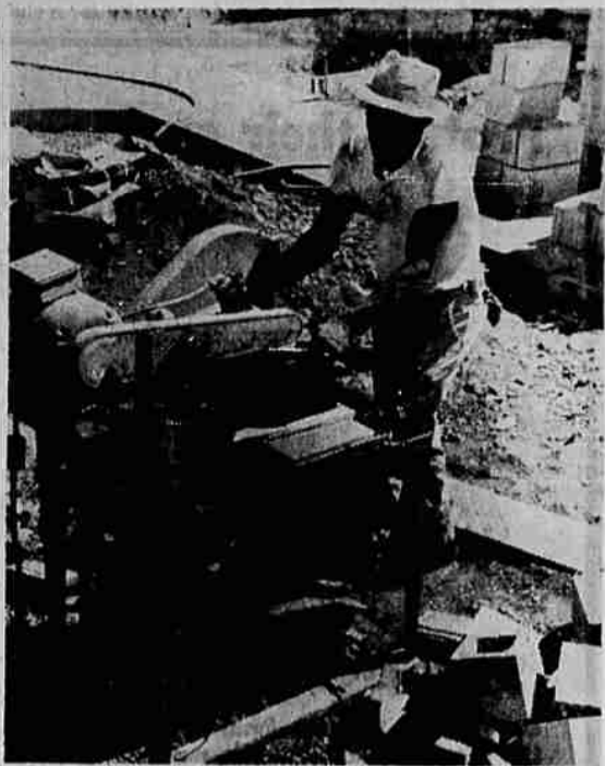
CUTTING BLOCK — A workman is shown above cutting block which will be used in the addition to Phoenix High school. The addition is expected to handle students who formerly attended Talent High school, which will be used as a junior high school in the consolidated district. Other renovations also have been done this summer in preparation for school opening.
