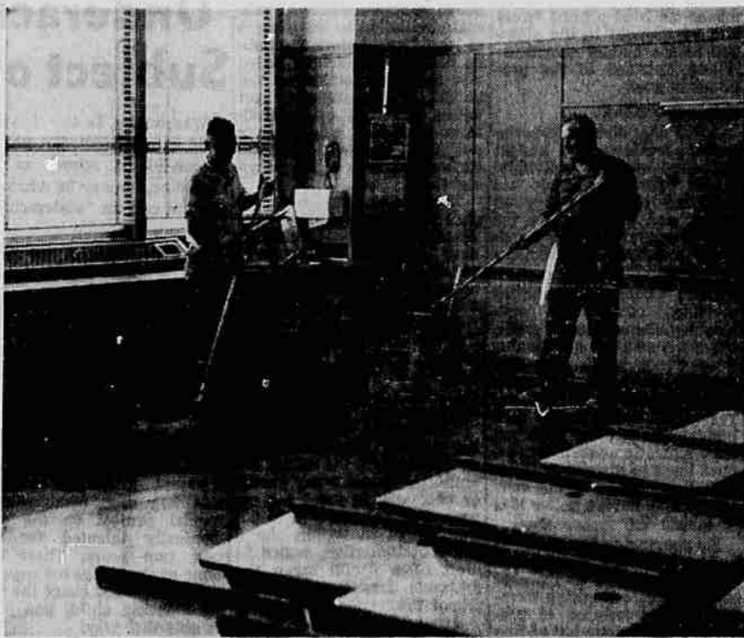
REFINISH FLOORS —One of the major projects in the Medford school district's summer program is refinishing all the floors in the district. Above Perry Strom, left,
