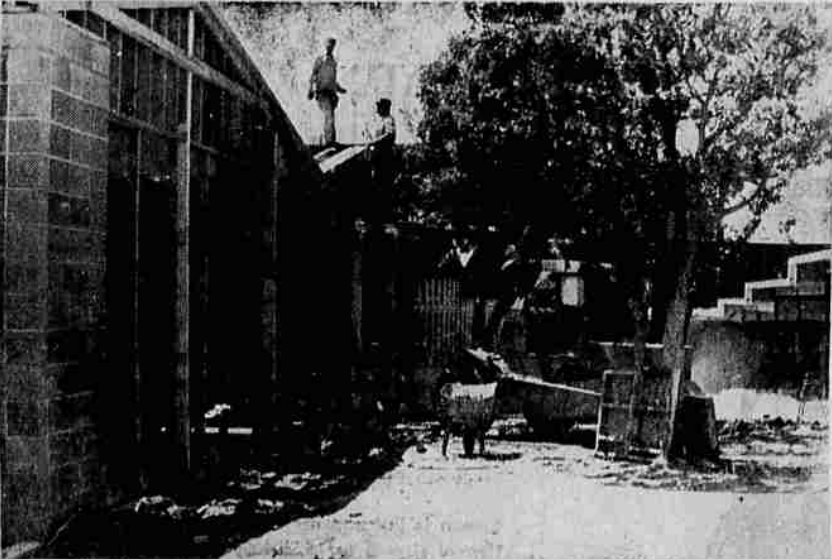
HOOVER ADDITION - New additions to Medford public schools includes this one under construction at Hoover school. Financed through a bond issue for a two-year building program, the additions will handle an anticipated increase of about 300 students in the district this fall. The additions are single wall construction - that is one wall serves two classrooms or both the interior and exterior.
