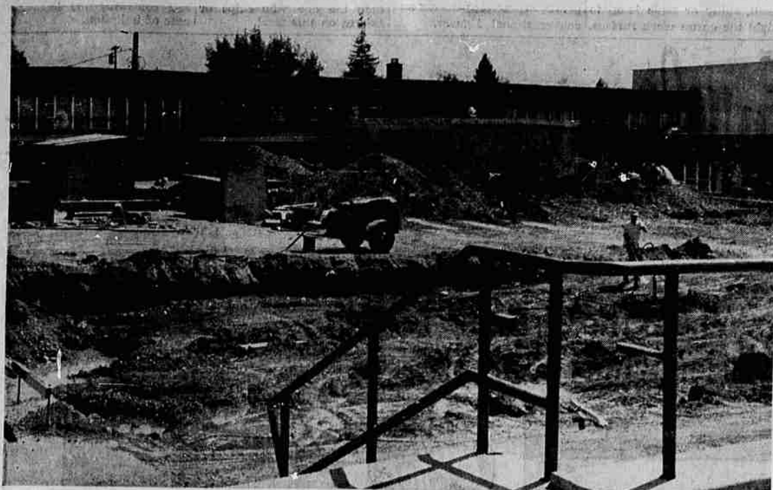
WORK STARTS - Work started last month on a six-classroom addition at Hedrick Junior High school, Medford. Batzer Construction company submitted the low bid of $127,492 for the project, which includes developing the courtyard in the center for planting. The addition is one of several in the Medford district.
