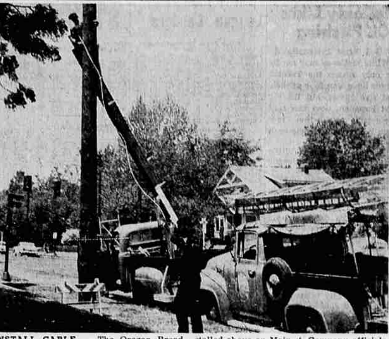
INSTALL CABLE - The Oregon Broadcasting company's distribution cable for television in Medford is shown being installed above on Main st. Company officials indicated house-to-house connections may be made within a few weeks.
