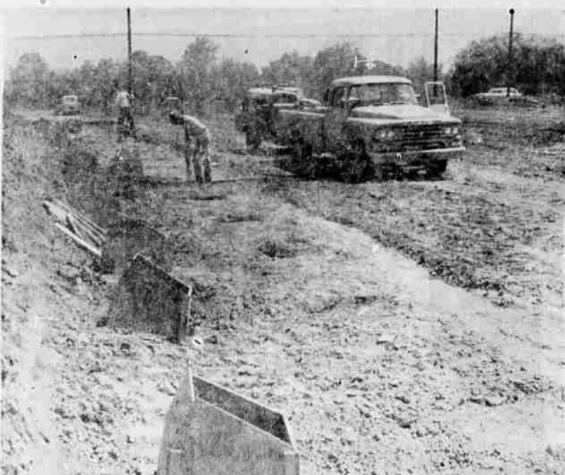
RINK SITE—Workmen above are shown as they prepare footings for the large laminated arches that will form the roof supports for the Jackson County Rollarama being built two miles south of Medford on Highway 99. The skating area of the 85x144 foot building will be floored with pecan veneer, one of the hardest commercial woods, according to Norris Porter, construction supervisor for Siskiyou Development company, contractors. The front of the structure will be built of Alpine logs, a product manufactured locally. The skating rink will be completed about mid-August, Porter said.
