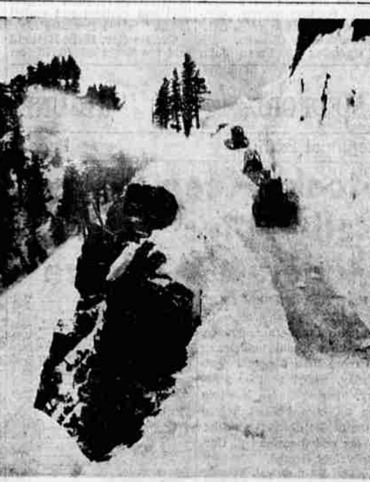
CLEARING ENTRANCE—Bulldozers and rotary snow plow are shown above clearing the rim road at Crater Lake National park so the north entrance road may be open by June 15. Heavy snowfall in April and May handicapped park crews in their efforts to clear the winter's snow from roads and
